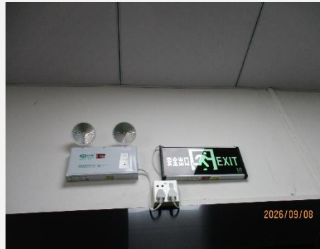
4-2: Emergency exit lights and exit sign
