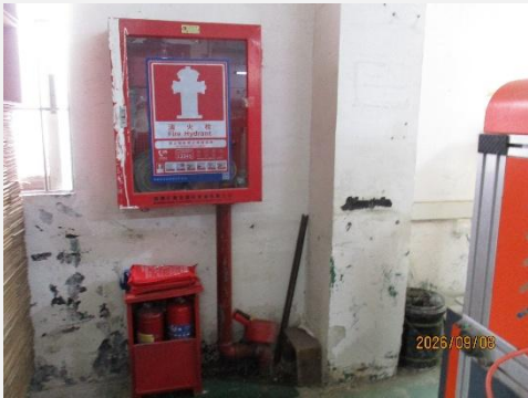
4-1: Fire extinguishers and hydrant
